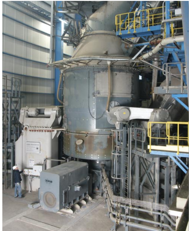
Figure 4: View of the MVR-R 3750 vertical roller mill grinding cement raw materials in the Lukavac cement plant in Bosnia-Herzegovina
