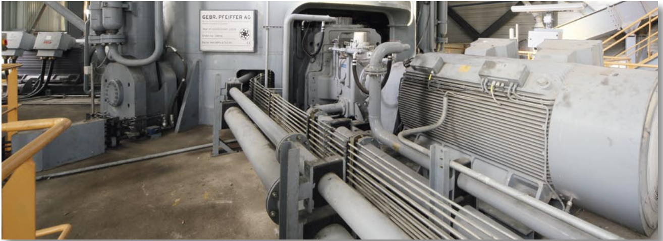
Figure 5: View of the first industrial MultiDrive with 3 x 1450 kW drive modules in an MPS 4750 BC vertical roller mill for grinding cement in the Val de Seine grinding plant in France
