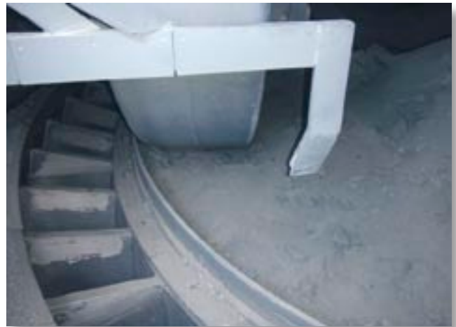
Figure 15: View of a grinding roller in the MVR 5600 C-4
