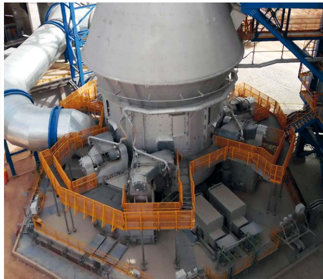
Figure 11: View of the drive situation for the MVR 6700 C-6 vertical roller mill at Biskra
