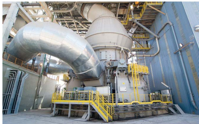
Figure 12: View of the drive situation for the MVR 6700 C-6 vertical roller mill at Barroso
