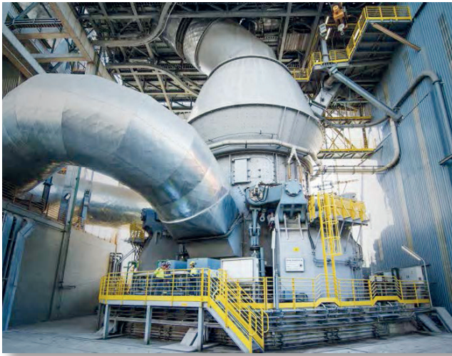
Figure 3: View of the cement mill MVR 6700 C-6 in Brazil
