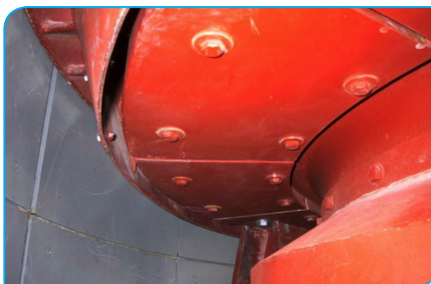
Left - Figure 3: Heat shield and thermal insulation for grinding bowl in hot gas channel.
