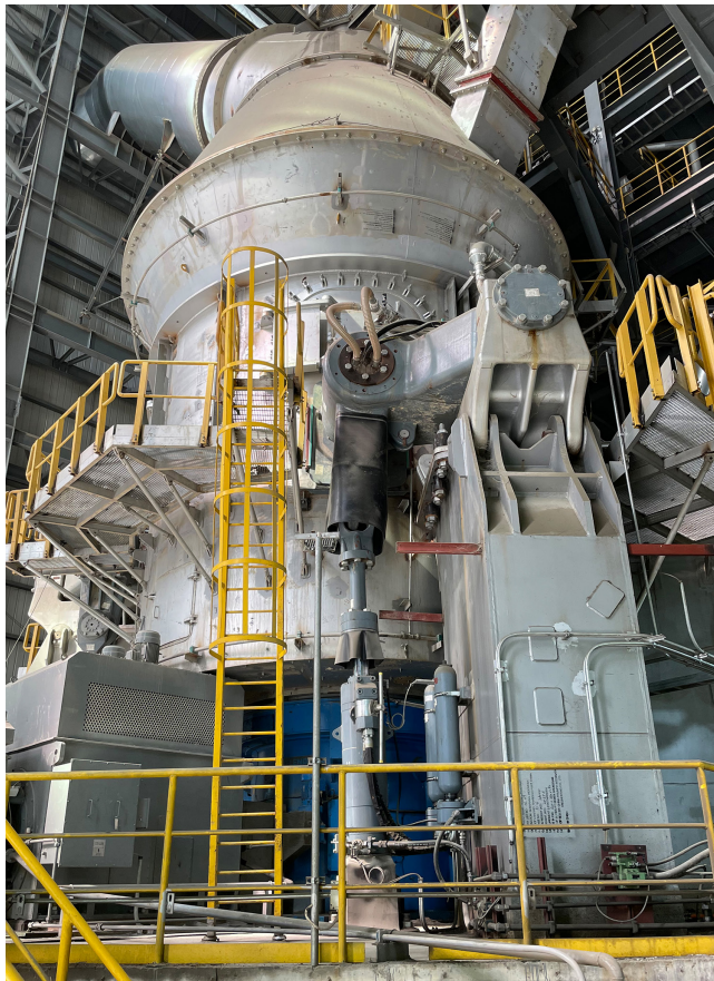
Figure 1. MVR vertical roller mill.
