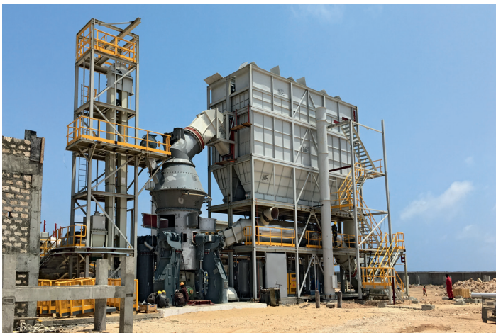
Figure 5. Mill with ancillaries, filter, and hot gas generator in Kenya.
