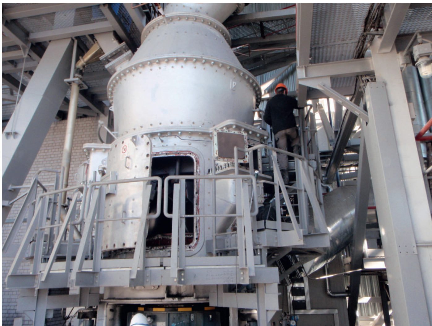
6 MPS 200 BK installed in the Ukraine
