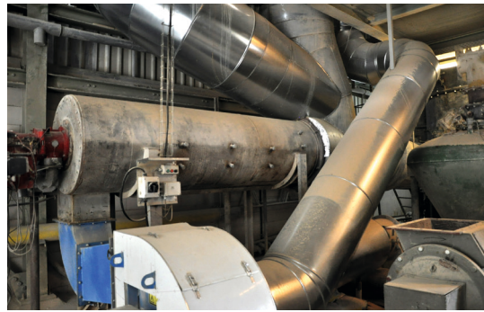
4 Hot gas generator from Gebr. Pfeiffer with new dilution air fan after the modifications of Steps 1 and 2
