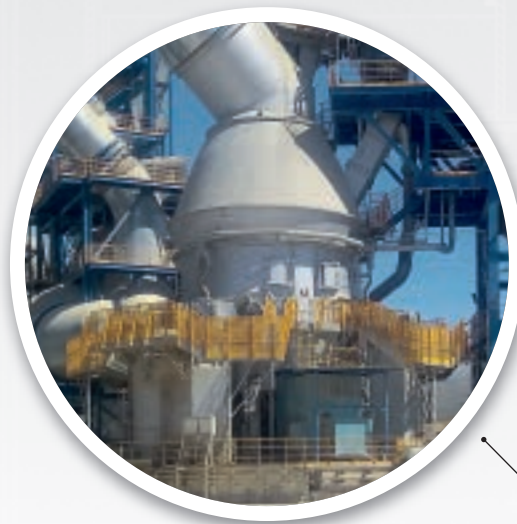
Cement raw material grinding with MVR vertical mills
