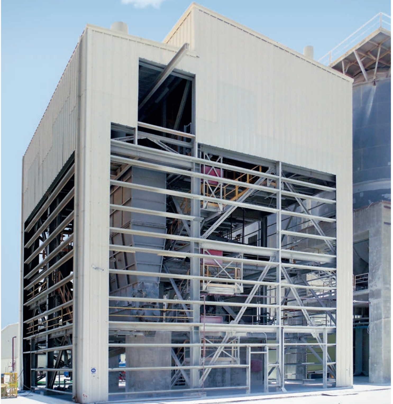
Lime hydrating plant in Saudi Arabia including SLV high-efficiency separator , MRD ball mill and KLV lime hydrator
