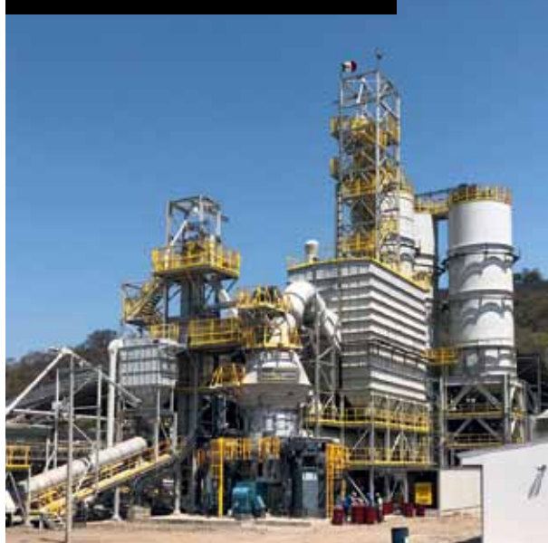
The grinding area of the ready2grind facility
