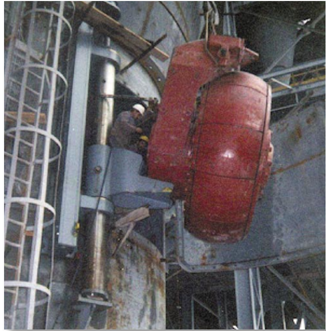
Figure 3: View of the MPS Lift and Swing system
